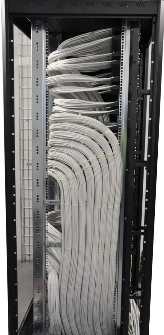
Patchpanels installed in 19" rack – side view
